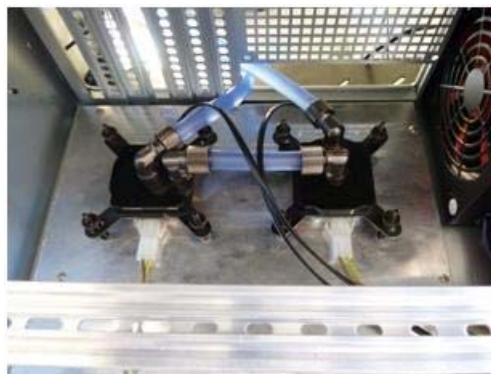
Figure 7. Dummy heat-loads inside a server case.
